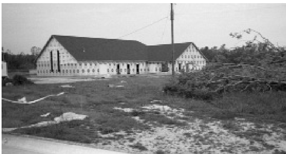
Construction progresses on the new home of Mount Zion United Methodist Church.
